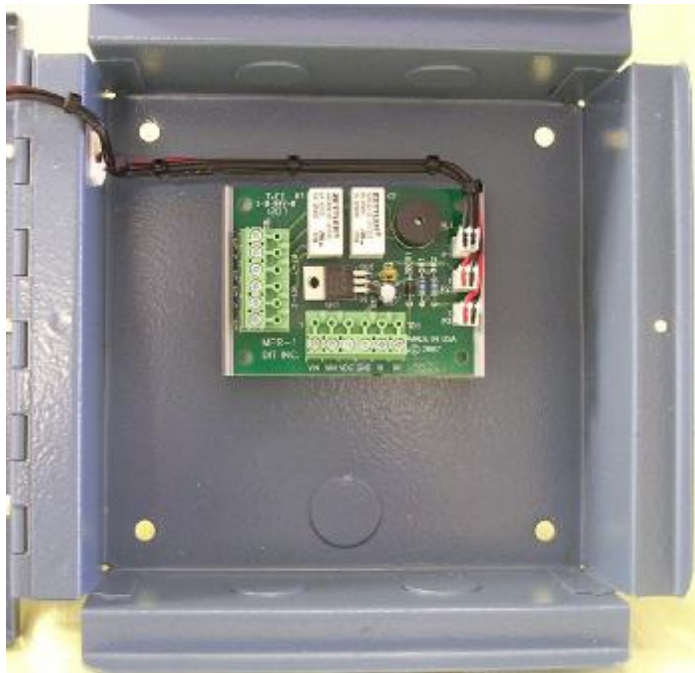
MPR-1 Alarm Board
